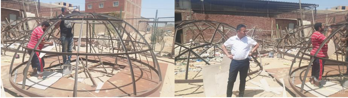
Shape 26 clarifies constructional sectors of the iron segments for the first dome
