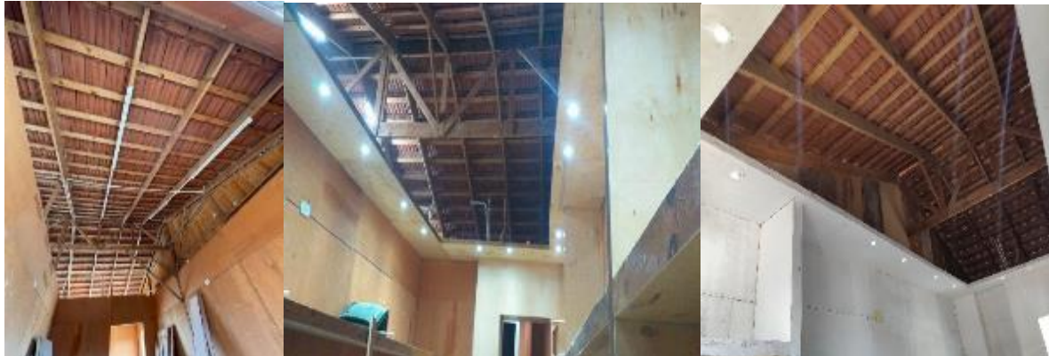
Photos n. (20) show the development of the ceiling before and after, the last one for the ceiling with lighting and initial paint.
