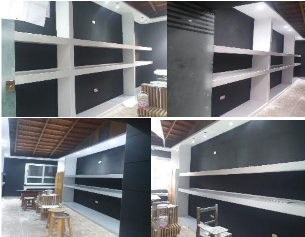
Photos n. (27) show wall CC` and wall AA` after the paint process.
