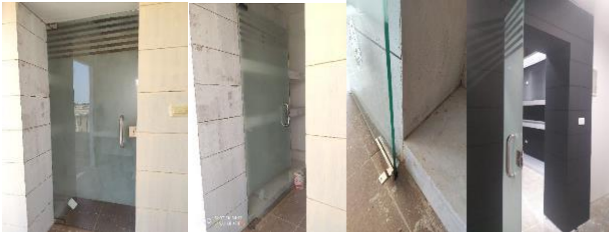
Photos n. (24) show a close shot of the wall EE` after fitting the glass door and the last one after the paint stage.
