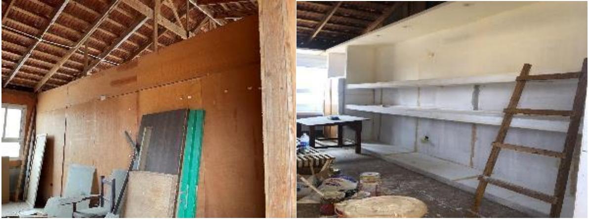
Photos n. (15) show the wall AA` before and after fixing the shelves that will carry the displayed pieces of furniture, the storage unit, and the desk. The second photo was in the fixing shelves stage.
