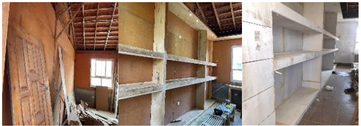
Photos n. (16) show the wall CC` before and after fixing the shelves.
