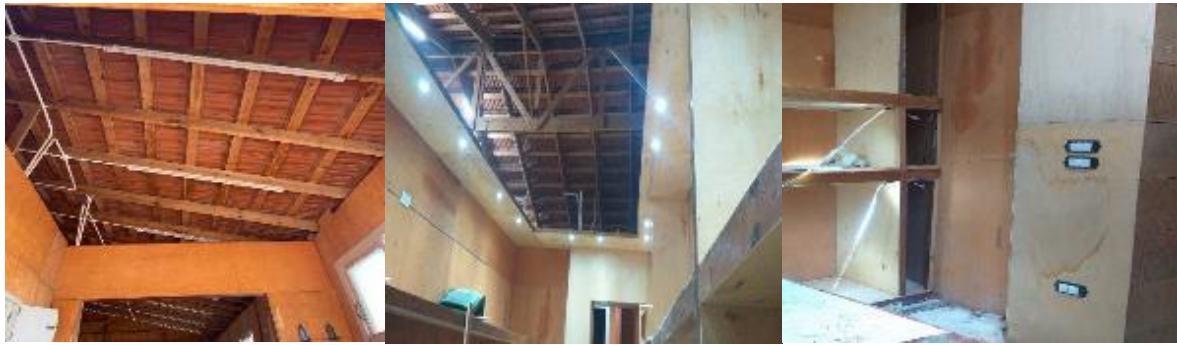
Photos n. (21) show the development of the lightning process, the electrical supply of the wires, and the installation of the final direct and indirect lighting and their electrical switches.
