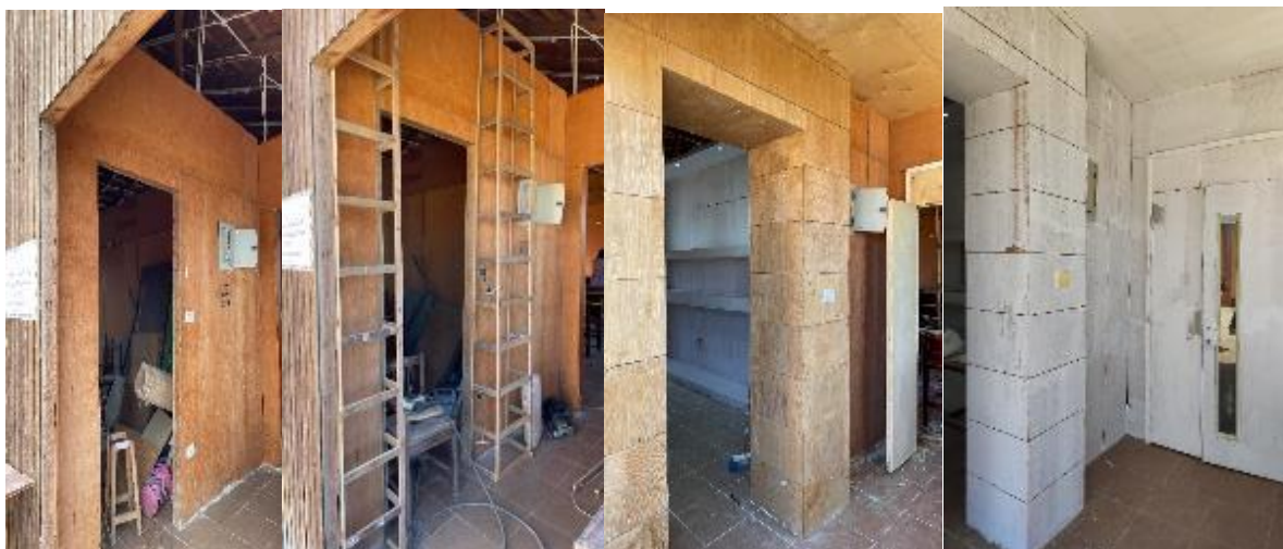
Photos n. (23) show the wall EE' before, though, and after fitting the wooden cladding. The last photo was in the initial paint stage.
