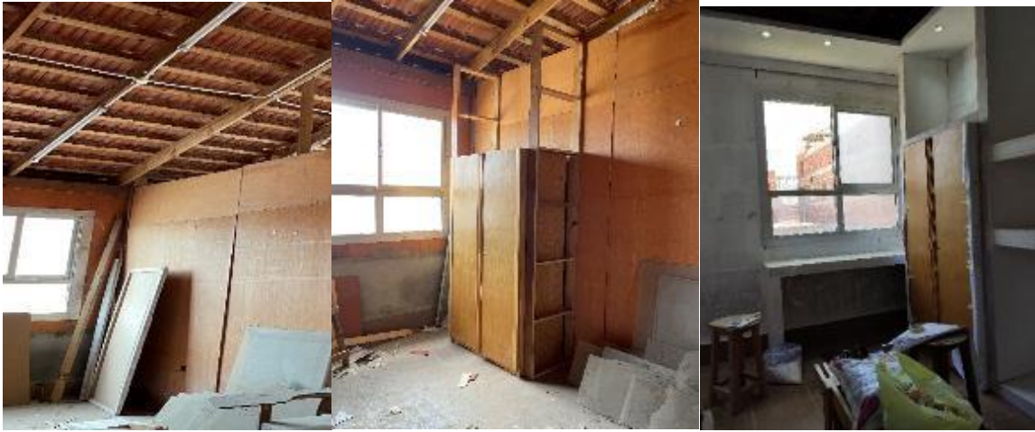
Photos n. (18) show the wall DD` and part of the wall AA` before and after fitting the storage unit, and the desk. The last photo was in the primary painting stage.
