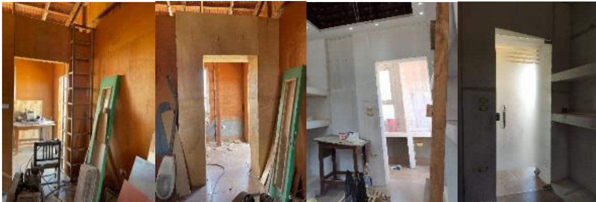
Photos n. (19) show the wall BB` before and after installing the wooden cladding, the initial paint stage, and after fixing the door.
