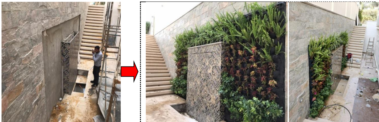
FIGURE 14: SHOWS A WALL THAT WAS IMPLEMENTED BEFORE AND AFTER THE INSTALLATION OF THE LIVING WALL IN THE HYDROPONICS GREEN WALL SYSTEMS. [28]
