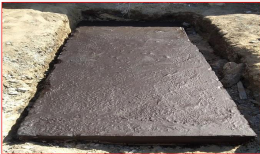
Fig (13). Shows the concrete and the dripping burlap placed on the bitumen material to protect the base from ground water
