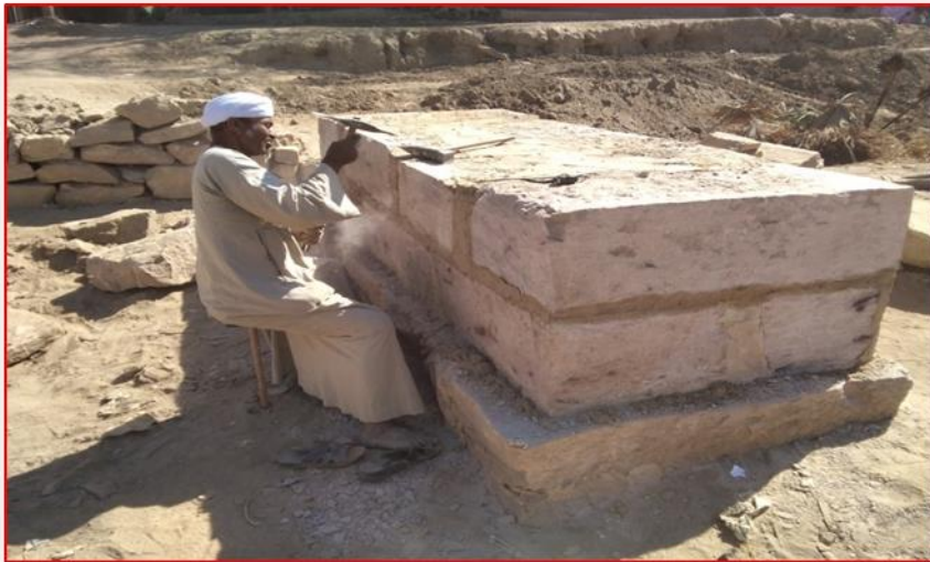
Fig (18). The shape of the first course, and the second after installation on the base and filling the gaps and joints between the stone blocks with mortar
