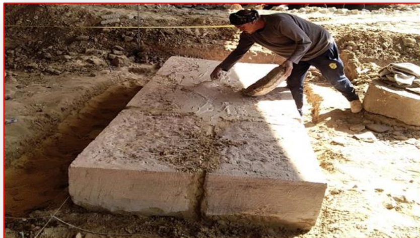
Fig (16). Placing the foundation course in the base and placing the mortar on it to connect it to the rest of the other courses
