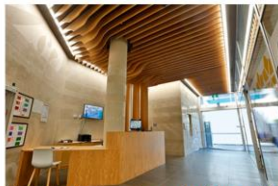
Picture No. (14) shows the use of wooden panels in the ceiling of the reception area in a psychiatric hospital:
